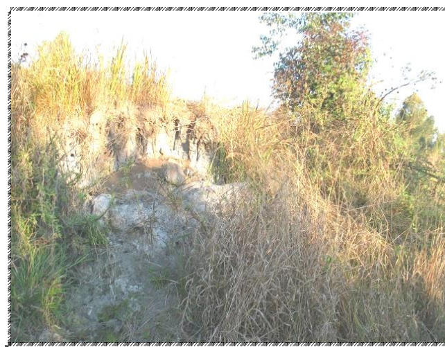
Figure 4.3: Signs of bank failure at Kuthindi site
